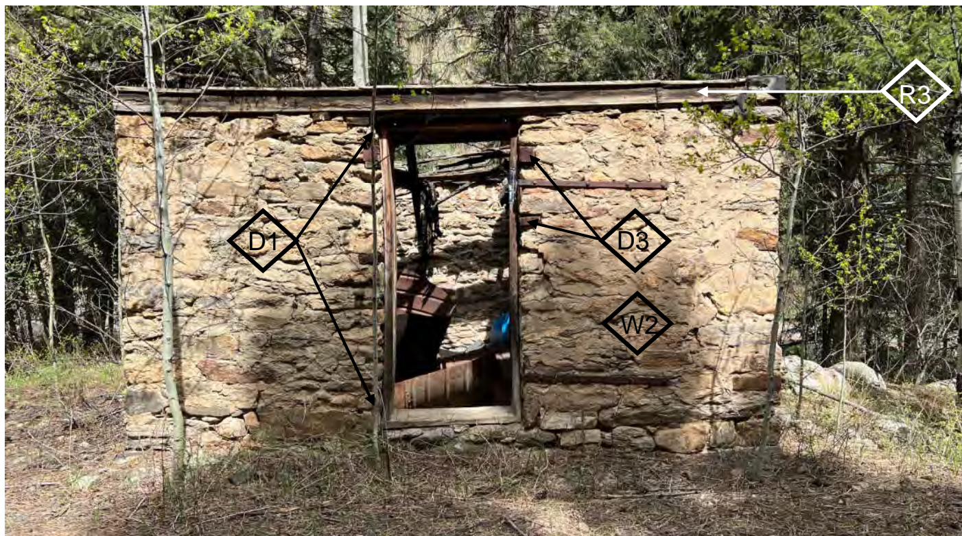
7. Main East Elevation - Original steel plate door is missing (May 2024)
