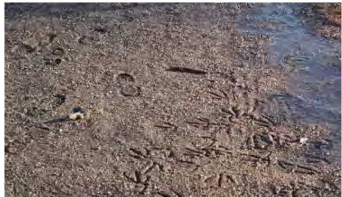
Water running down the slope gathers on the crusher fines trail because of insufficient cross slope of the trail.
