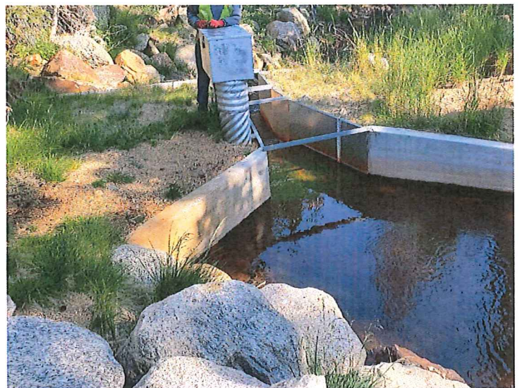
Photo 10 - Outlet flume and dry seep location on left
