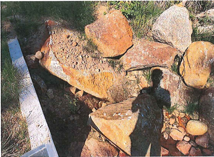
Photo 5 - Seep downstream of flume wingwall
