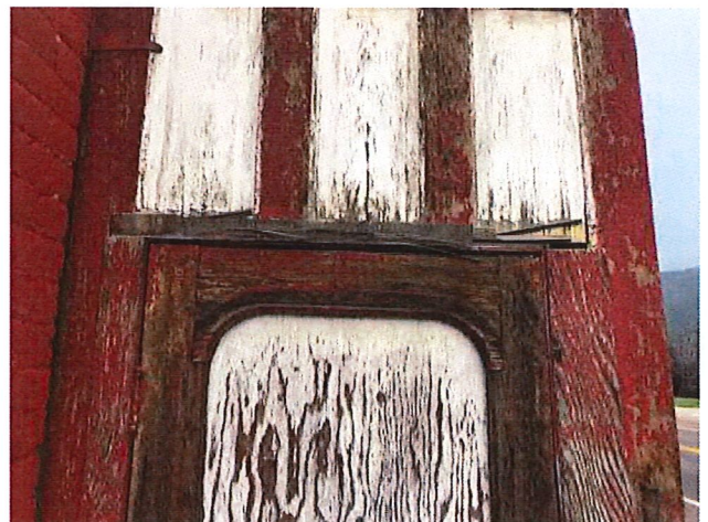
Photo 3 (Above): The door frame member that was added at the head of the man door is mostly missing. The door frame jambs are simple 1x wood members.
