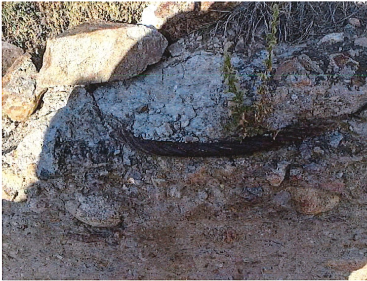
Exposed steel cable reinforcement
