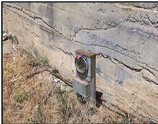
Typical utility hook-up in Lots 3-9. Some non-functional.
