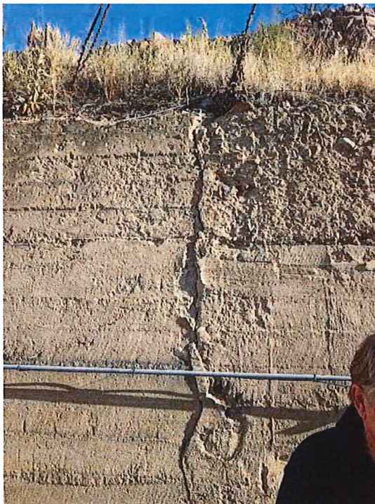
Exposed aggregate and cracking in in concrete retaining wall
