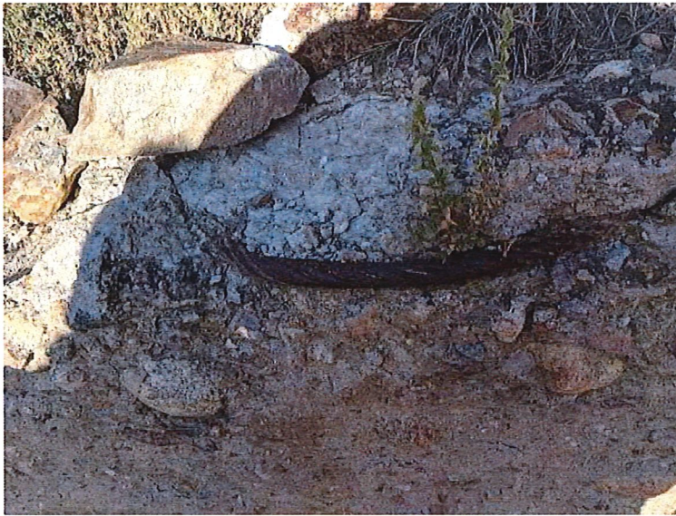
Exposed steel cable reinforcement
