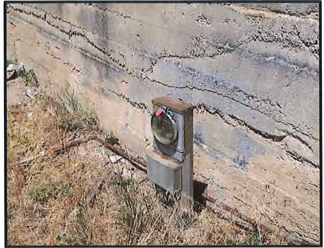
Typical utility hook-up in Lots 3-9. Some non-functional.
