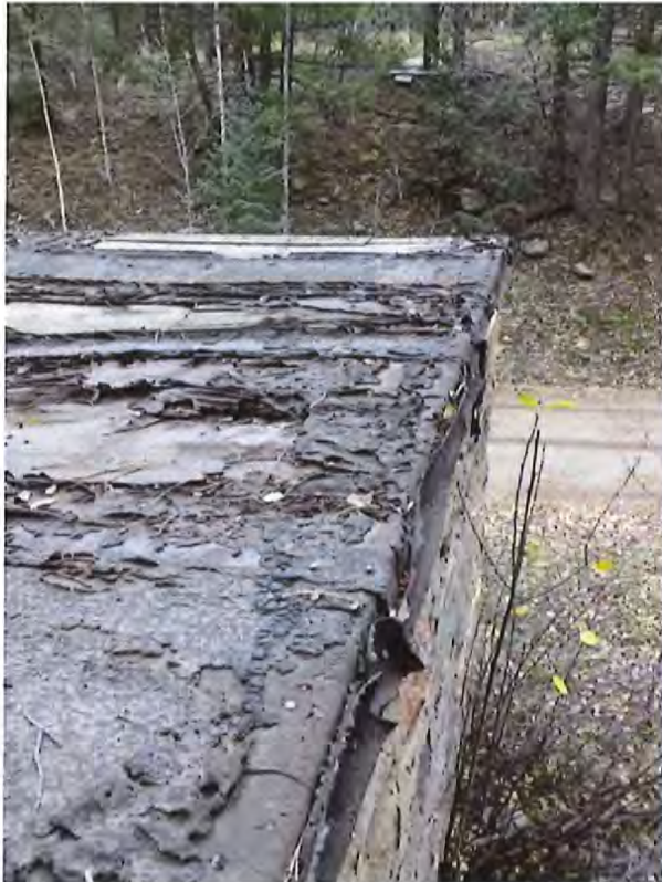
Figure III-15. There are approximately two layers of existing bituminous sheet roofing, seen in this view of the south side of the powder house looking east. The underlying wood sheathing boards are exposed to the weather in many locations.
