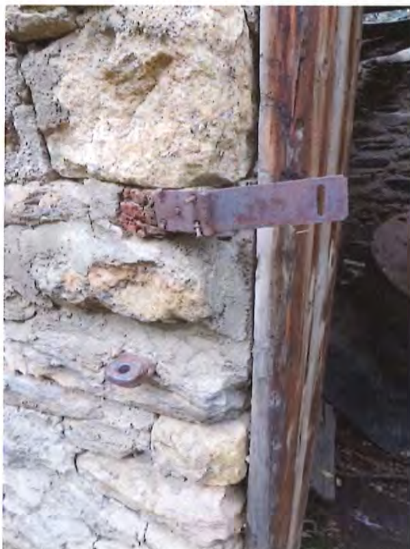
Figure III-21. The steel hasp and eye for securing the door remain installed in the wall. The screws holding the hasp are loosely attached to the wood buck while the eye was laid in the stone rubble wall. The door frame is chipped.
