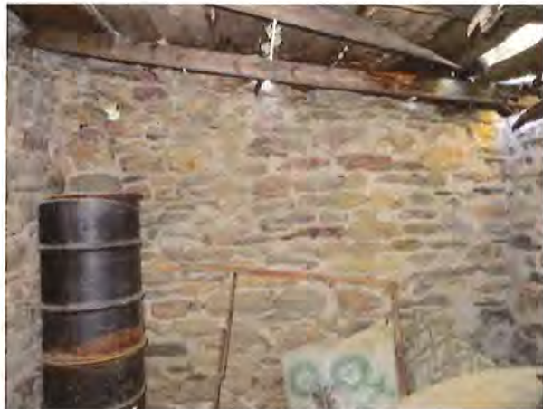
Figure III-24. The finish of the interior walls is the same as that of the exterior walls, which is random or uncoursed stone rubble laid in mortar. A broken and missing roof rafter can be seen in this view looking towards the southwest corner of the room.
