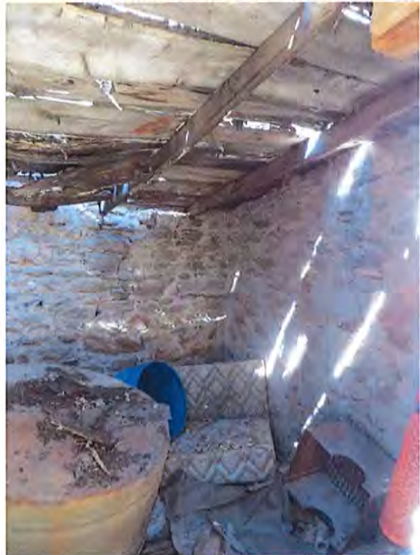
Figure III-27. With its entry door missing, the Powder House has most recently been used as a household refuse deposit location. Large barrels, automobile parts, and furniture fill the interior space. A crack is developing in the west wall where moisture has entered the top of the wall.
