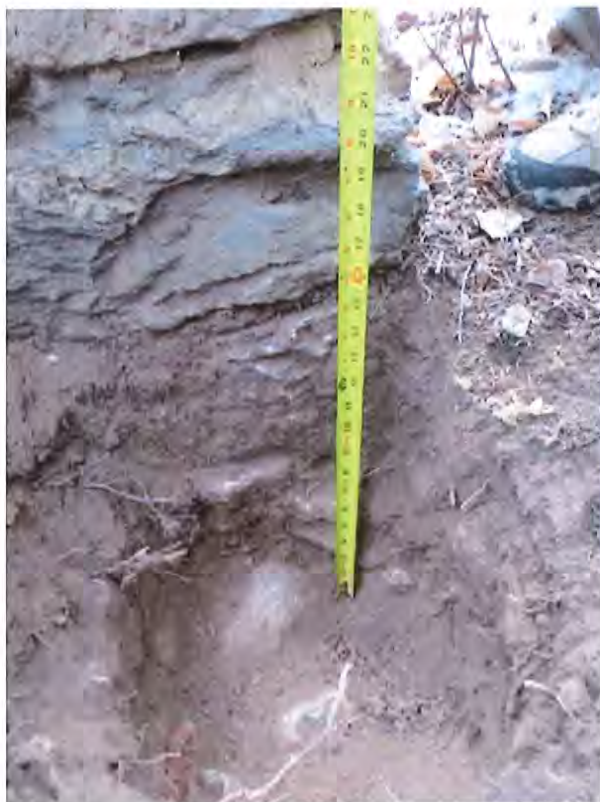
Figure III-4. The foundation walls extend above grade to function as the powder house's exterior walls. Large boulders, which function as footings, can be seen at the bottom of the excavation. Large gaps can be seen between the stones where mortar is missing.
