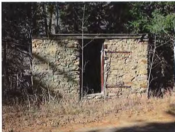
Figure III-17. The main entry door is missing at the east wall of the Powder House. The wood door frame and portions of the steel strap hinges remain.
