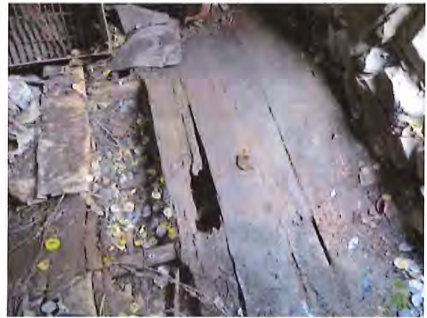
Figure III-25. The flooring is cracked, broken, and missing. Portions of the supporting wood floor joists are exposed to view and deteriorated from exposure to moisture.
