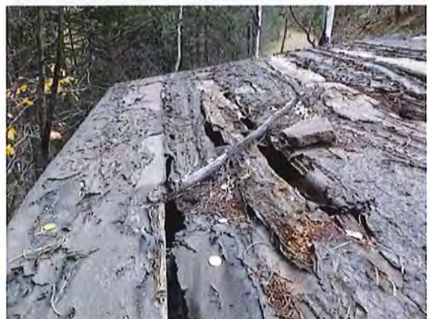
Figure III-14. The bituminous sheet roofing is mostly missing, resulting in much of the wood sheathing boards being cracked and missing from exposure to the weather.
