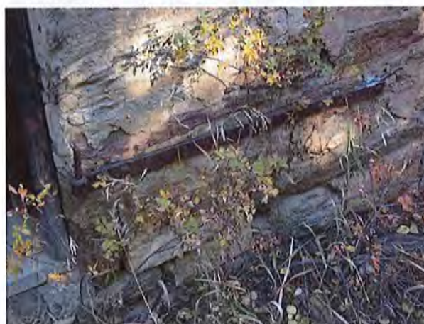
Figure III-19. The former entry door's two steel strap hinges remain attached to the east wall. The lowest strap hinge is visible in this view looking towards the door threshold.
