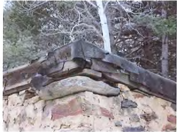
Figure III-16. Portions of the east wood fascia board and the north wood rafter are visible in this view of the northeast corner of the roof. The deterioration of the roofing system has allowed moisture to enter the top of the perimeter stone walls. Mortar is now missing in some locations, including the top of the northeast corner where a stone appears to be ready to fall out of the wall.
