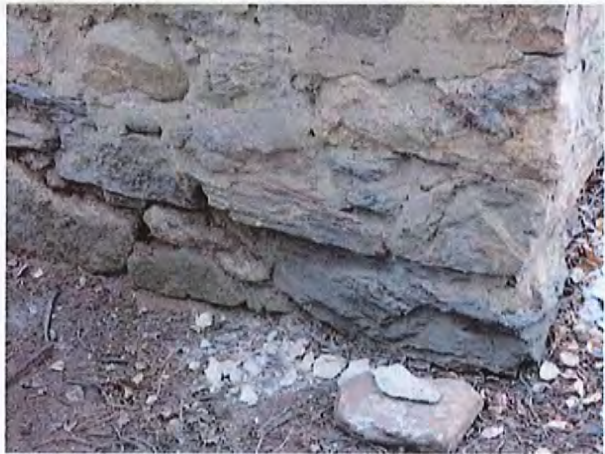
Figure IV-2. Much of the mortar has fallen out of joints at the bottom of the exterior walls. The original mortar should be tested to determine its mix for masonry repairs at the powder house.
