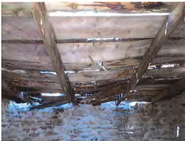
Figure III-5. The four interior roof rafters can be seen in this view looking west. The second rafter from the left side of this view is partially missing.
