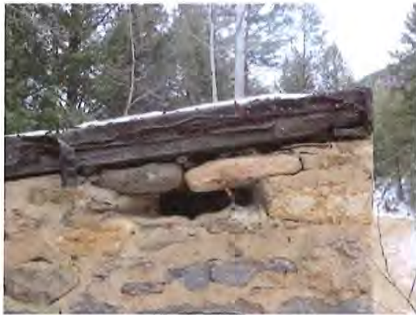
Figure III-7. The roof rafters at the north and south ends of the roof edge are cracked, dry, and missing wood from their lack of protection from the weather. The south rafter is visible in this view of the top of the south stone wall; much of the bituminous sheet roofing that wrapped over the vertical faces of the roof is now missing. A wall opening was intentionally provided for ventilation; most of the screen is now missing.
