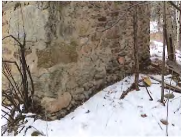
Figure III-10. Large stone rubble was utilized at the northwest corner of the building. The mortar joints at the bottom of the west wall are mostly missing from exposure to moisture. Consequently, some of the stones have fallen out of the wall.
