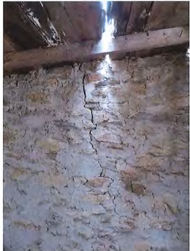
Figure III-9. The interior side of the north wall has been patched with mortar, in response to repairing the crack. The patching mortar is whiter and finer in texture than the original, suggesting a high percentage of Portland cement.
