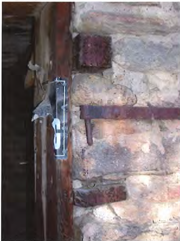
Figure III-11. The wood bucks appear to have been previously painted although they may be stained from a former rusty door.
