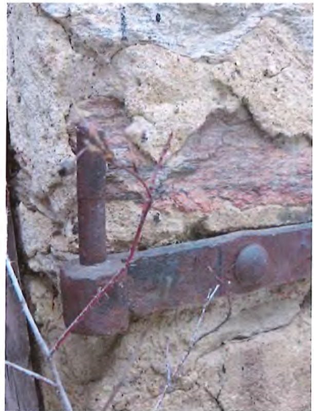
Figure III-22. Portions of the hinge pins remain attached to the steel strap hinges. The top half of the hinge pin once held the missing half of the hinge that was attached to the entry door.
