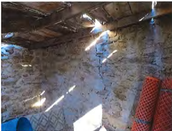
Figure III-26. Daylight illuminates a crack in the north wall, which is the result of moisture entering the top of the wall from a failing roof assembly.
