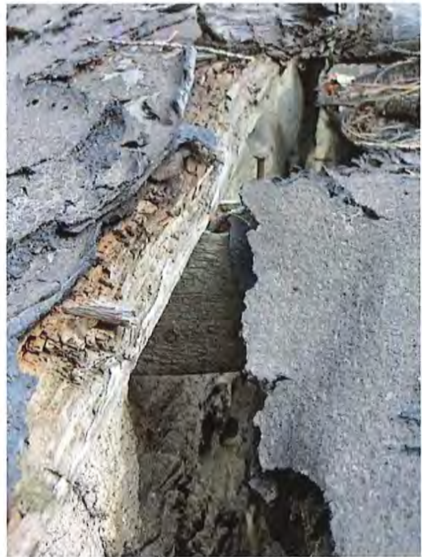
Figure III-6. A portion of one of the roof rafters can be seen where both the bituminous sheet roofing and sheathing are missing. The rafter is cracked and dry. Wood is missing along its top horizontal face.
