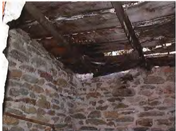
Figure III-13. The wood roof rafters and wood sheathing boards are exposed to view inside the powder house. Portions of the bituminous sheet roofing and wood sheathing boards are now missing due to moisture infiltration.
