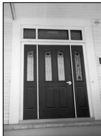
LEFT: Inappropriate replacement entrance.
