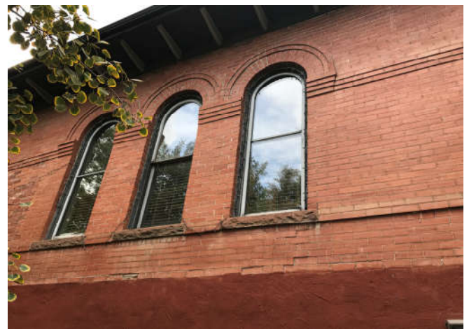
Figure 3. Existing cracked and damaged bricks on the front elevation.
