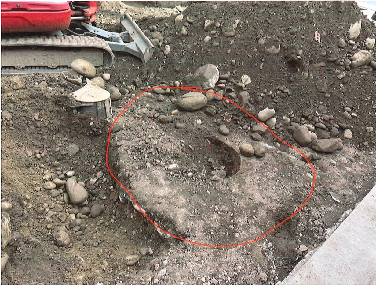
#002 - Existing Chunks of concrete in West Drive through.
