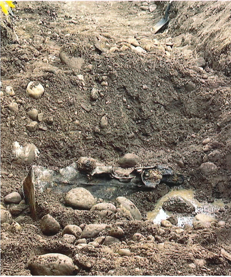
#005 - abandoned metal container. Possible soil contaminants.
