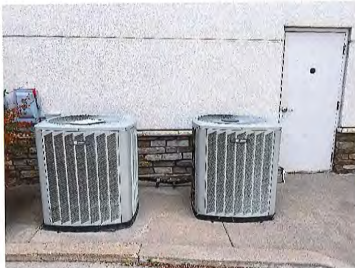
Figure 1: Condensing units on west side of building.
