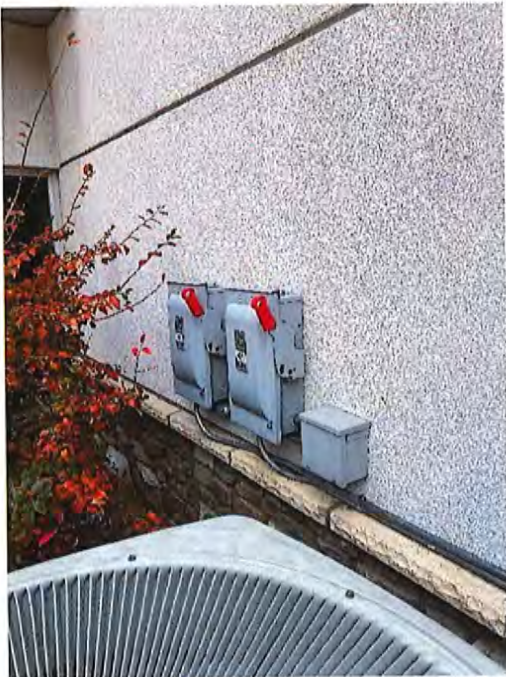
Figure 2: Condensing unit electrical disconnects. 240V-60A fused disconnects.
