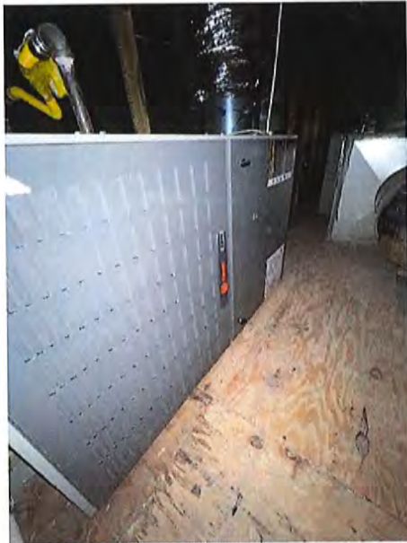
Figure 5: Trane XR80 gas furnace unit.
