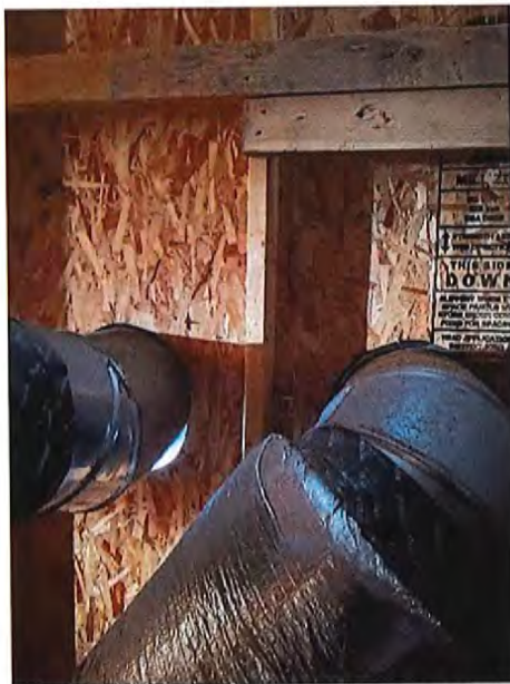
Figure 6: Fresh air intake penetrations. Fresh air intakes connect to return air on each furnace unit and are balance via a manual volume damper.
