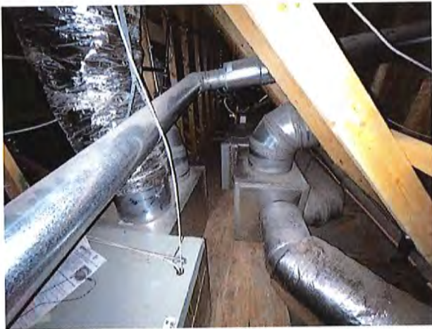
Figure 4: Furnace units ground mounted on walkway in attic.
