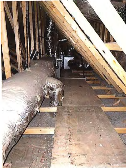
Figure 3: Walkway to furnace units in attic.
