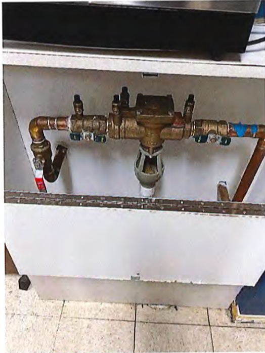
Figure 10: 1" Backflow preventer in kitchen.
