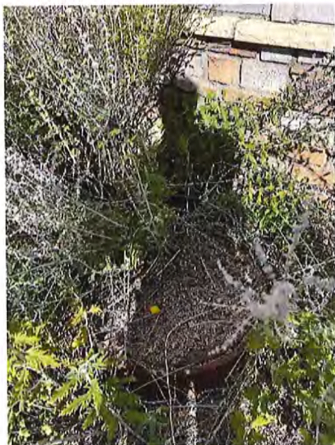
Figure 9: Domestic water meter on southside of building.
