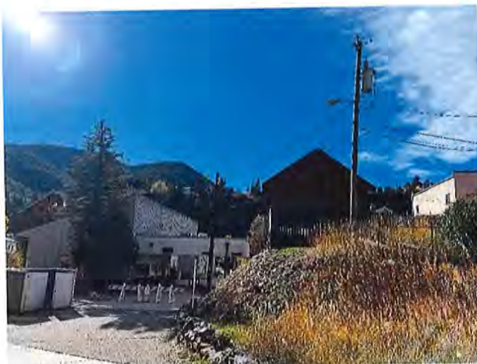
Figure 14: Pole-Mounted transformer servicing building.
