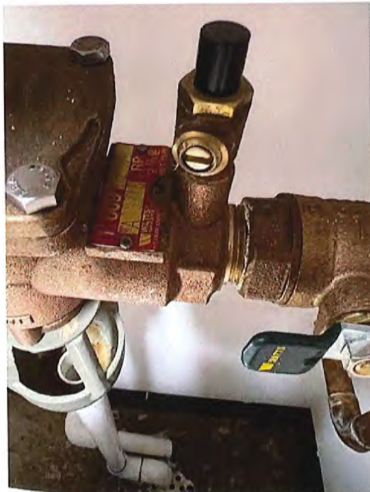
Figure 11: Floor drain below backflow preventer for condensate, water heater drain pan, and backflow preventer drain.
