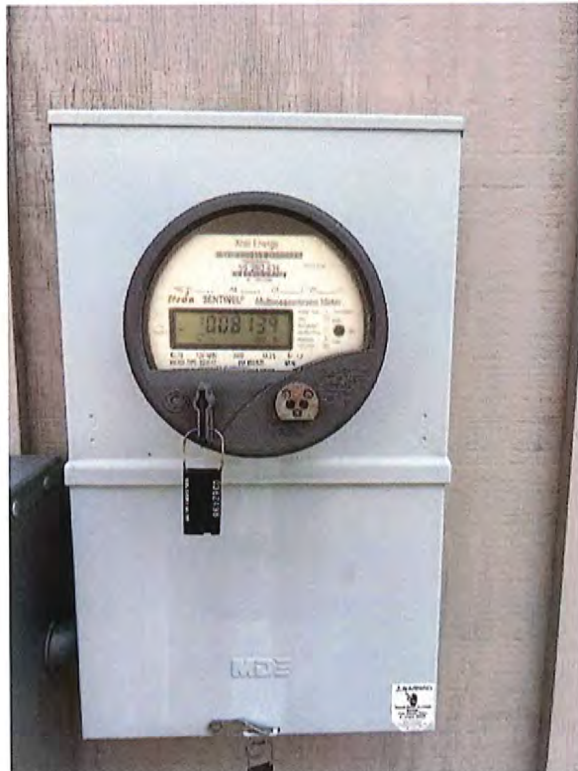
Figure 15: Excel Energy CL20 Meter. Meter# 59980434
