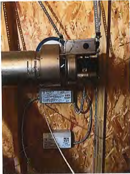
Figure 7: Power flue exhaust fan that assists in the combined B-vent system for the furnace units.
