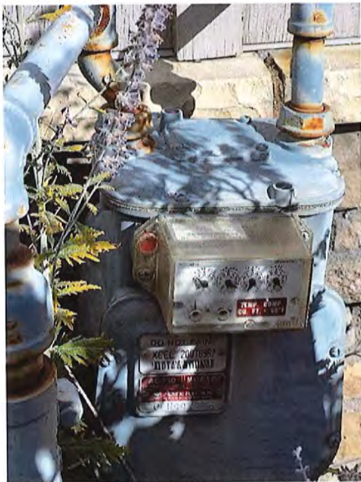
Figure 13: Gas meter on southside of building.
