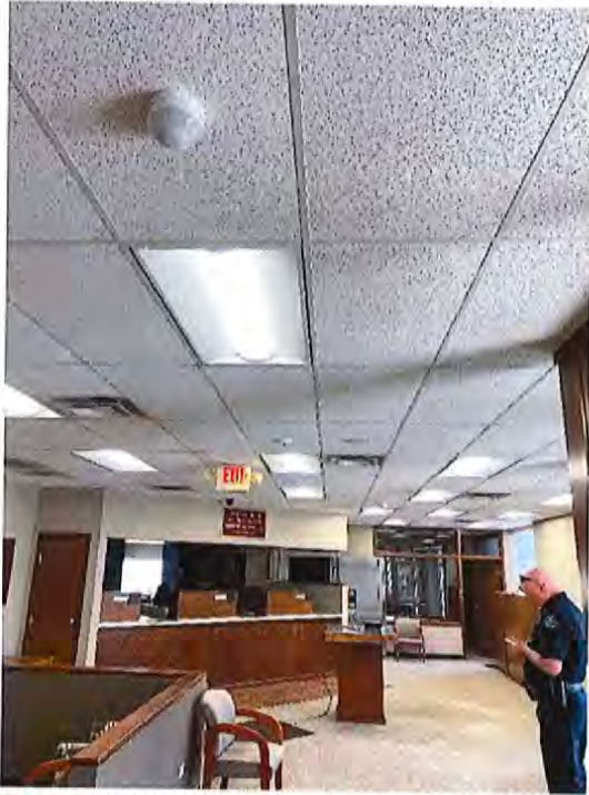
Figure 20: LED troffers in main lobby area.
