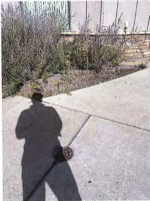
Figure 8: Curb stop for domestic water service on southside of building.
