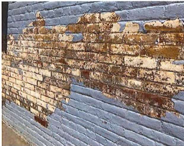
West wall – there are 2 spots like this.
